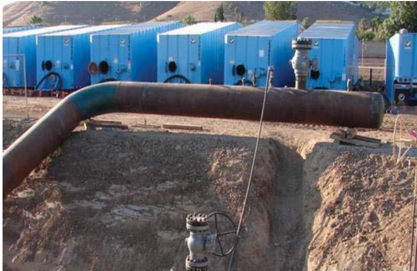
Figure 26: Water Tanks and Test Head
